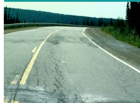
Rural roadway patched and uneven due to lack of maintenance and repairs.
