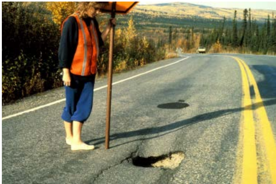
Roadway damage resulting from thawing permafrost. Photo by Thomas Kinney
