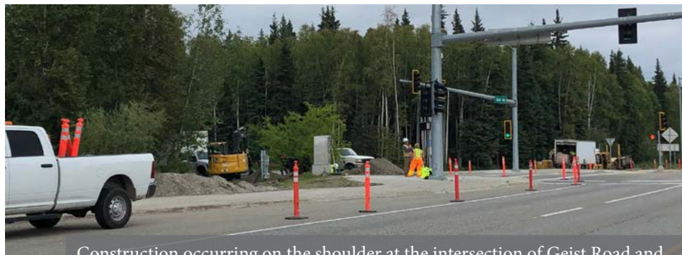
Construction occurring on the shoulder at the intersection of Geist Road and Thompson Drive in Fairbanks, Alaska during August 2021. Thompson Drive is a primary access route to the University of Alaska Fairbanks.
